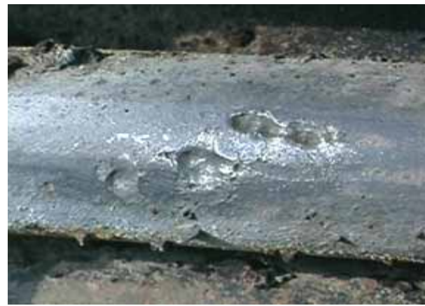
Tubel Fouling Deposit Tubercle Mud Pitting CORROSION
