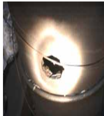
Radiant Bottom Manifold Erosion
